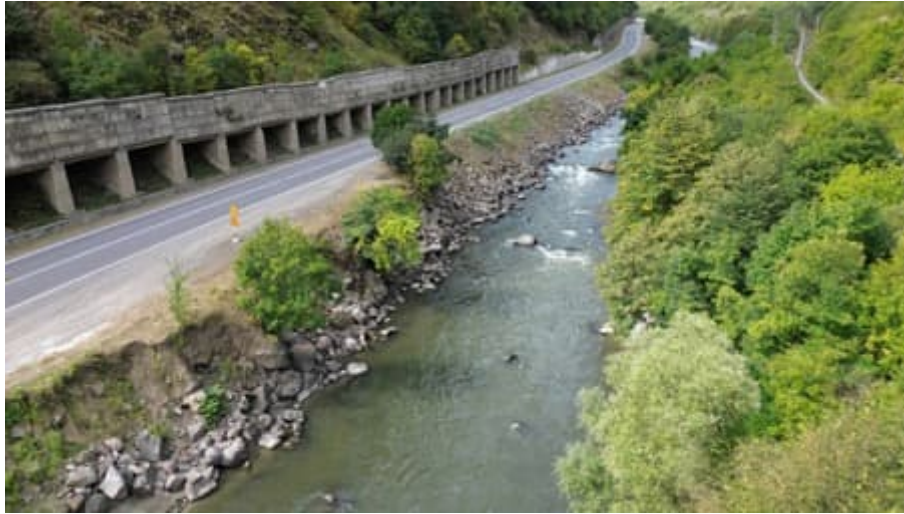
Figure 5: Drone photo of the river and road section with the buttress wall
